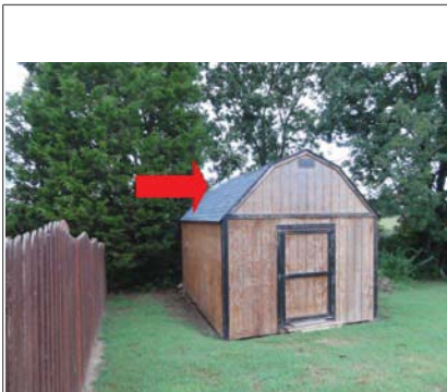
Roof needs repair
