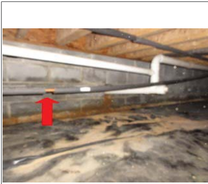
Sagging copper water pipe
