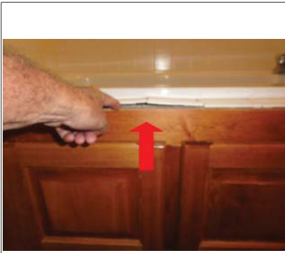
Tile pulling up
