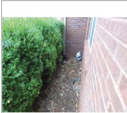
Left side of front porch that needs backfill
