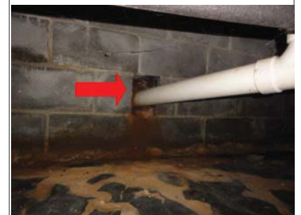
Drain entry PVC
