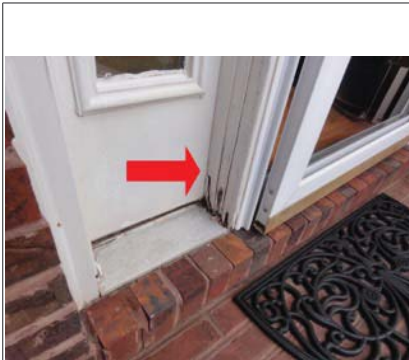
Door trim starting to rot
