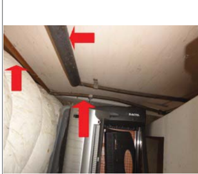
Plumbing pipes are not supported
