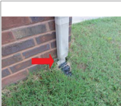
Gutter has separated
